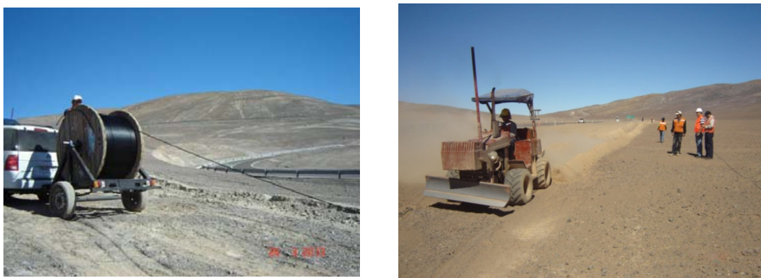
Figure 6. (Right) the fiber cable is directly installed in the trench that is then (left) filled back with excavation material that is then compacted.
