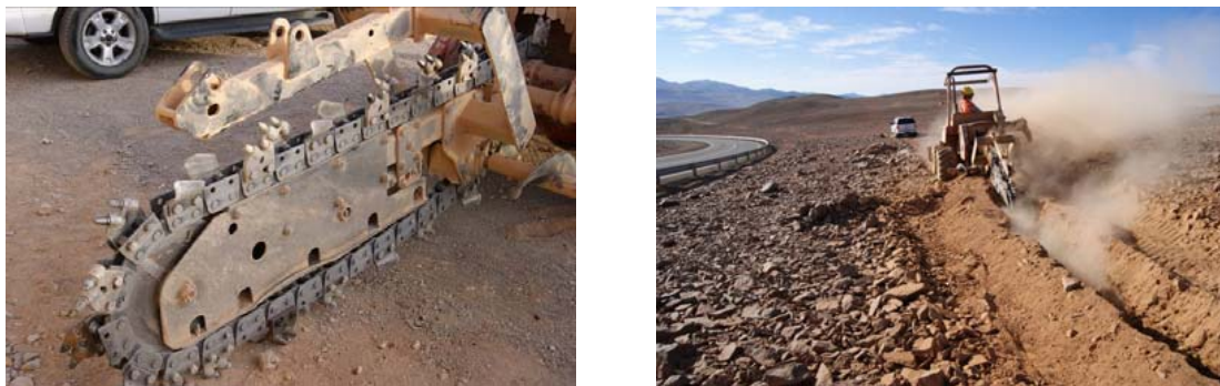
Figure 5. (Right) the cutting tool used to create the trench where the cable will be laid down and (left) the excavation.
